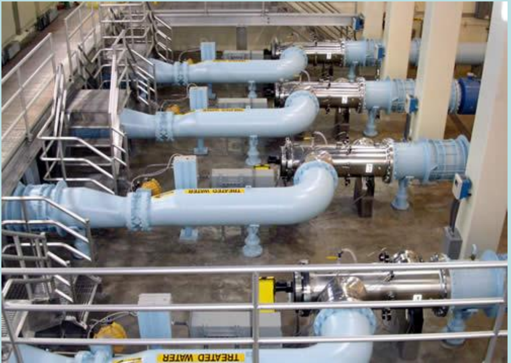
Drinking Water installation at the City of Henderson, Nevada
