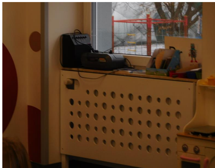
Figure 42 Convectors in classrooms
