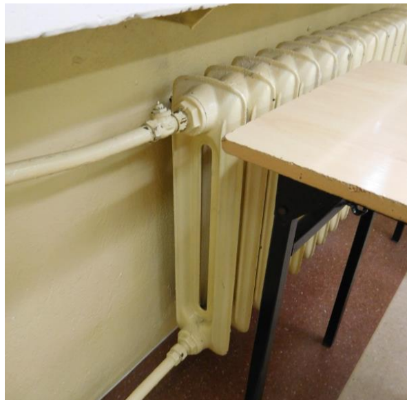
Figure 25 Iron ribbed convectors in classrooms
