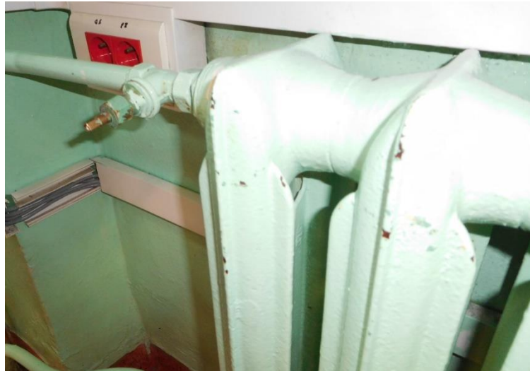
Figure 62 Iron ribbed convectors in classrooms
