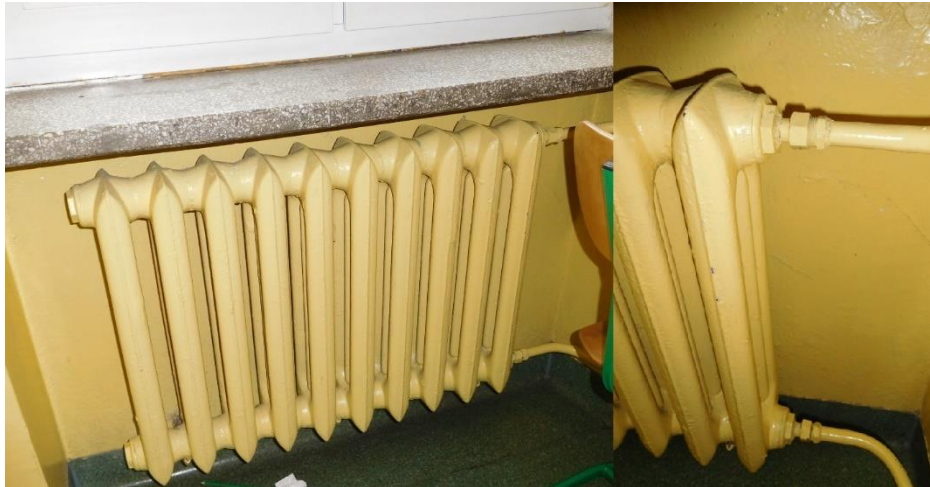
Figure 52 Iron ribbed convectors in classrooms
