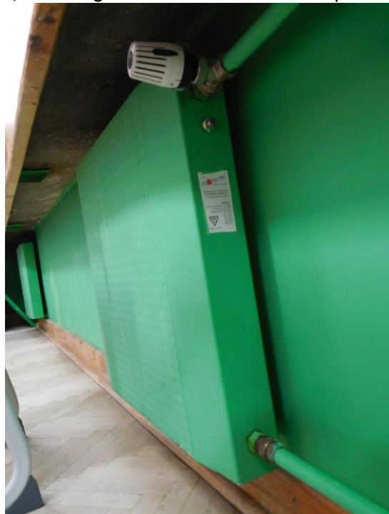
Figure 17 Convectors in classrooms
