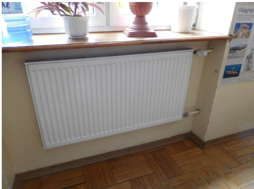
Figure 73 Convectors in classrooms
