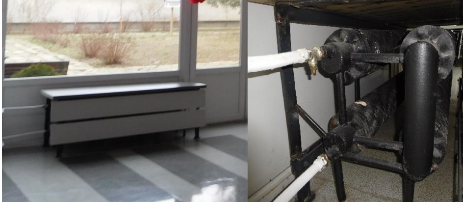
Figure 24 Pipe heaters in the corridors
