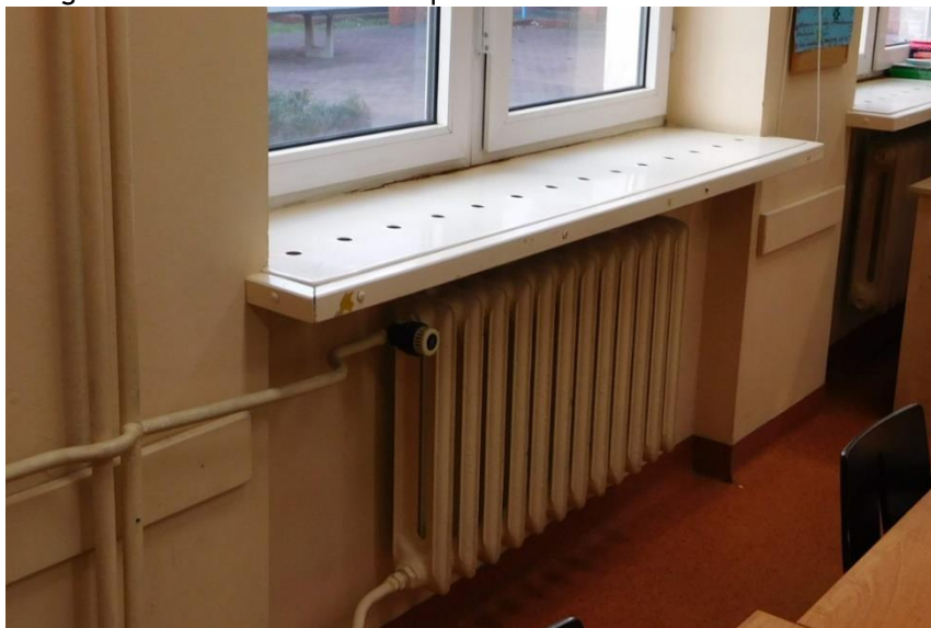
Figure 36 Convectors in classrooms
