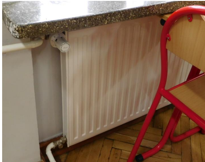
Figure 5 Convectors in classrooms
