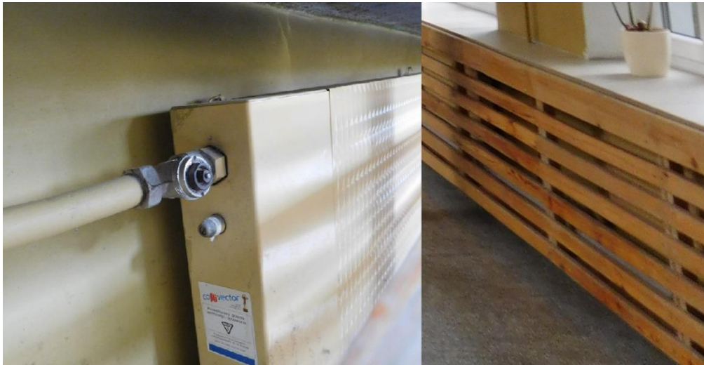
Figure 16 Plate heaters in the building
