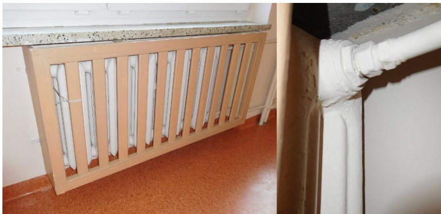
Figure 61 Iron ribbed convectors in corridors
