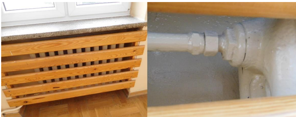
Figure 51 Iron ribbed convectors in corridors
