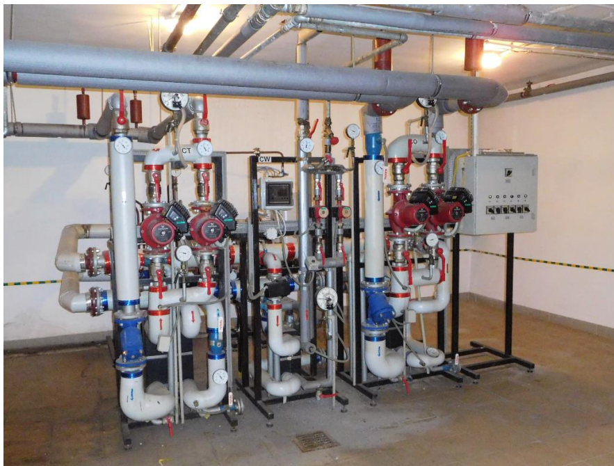
Figure 70 The heating source in the building
