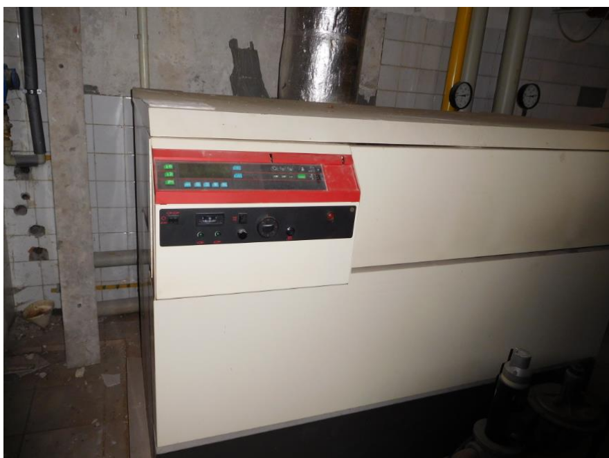
Figure 43 Heating source in the building
