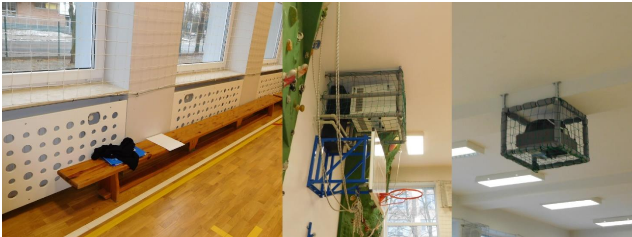
Figure 46 Thermal control devices in the sport hall
