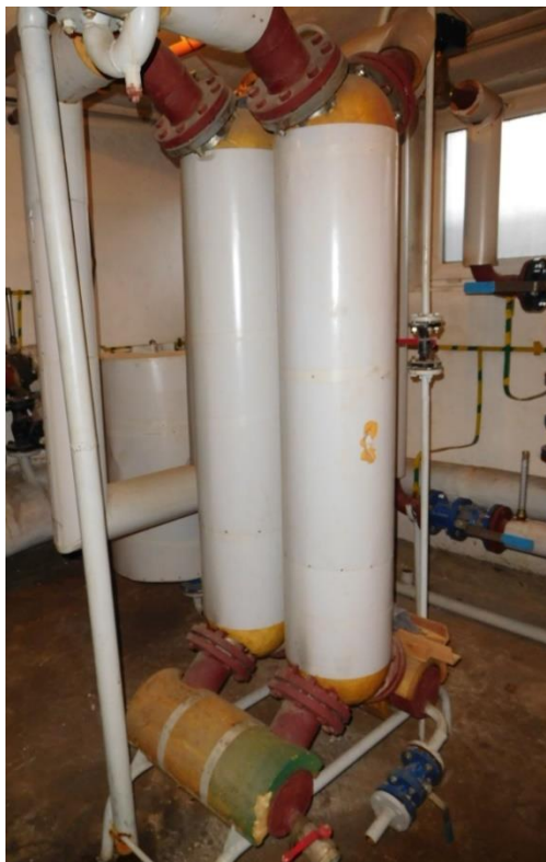
Figure 65 Heating source in the building
