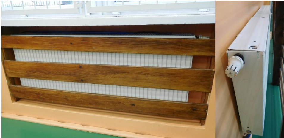
Figure 57 Plate heaters in the sport hall with thermostats
