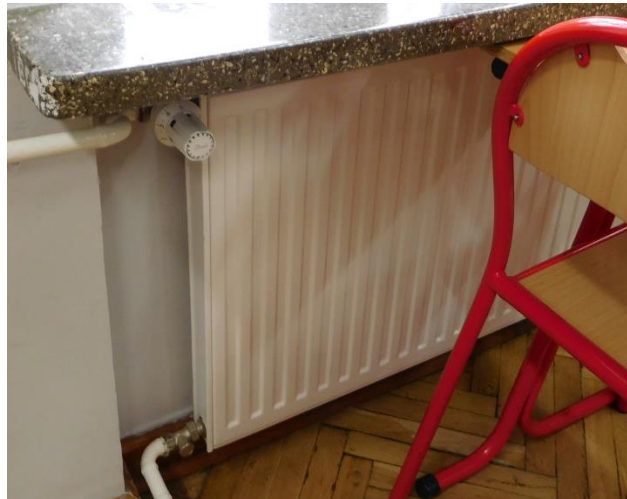
Figure 5 Convectors in classrooms
