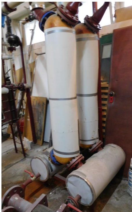
Figure 16 Heating source in the building
