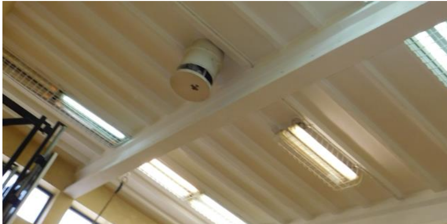
Figure 69 Sport hall ventilation
