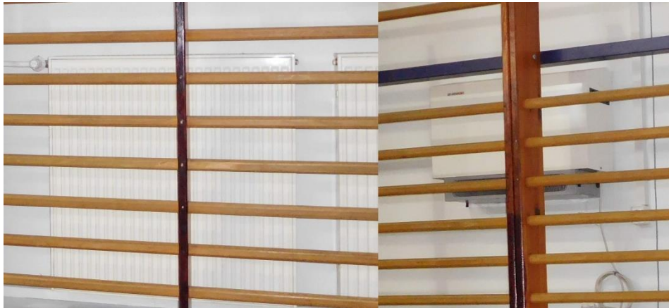
Figure 40 Thermal control devices in the sport hall
