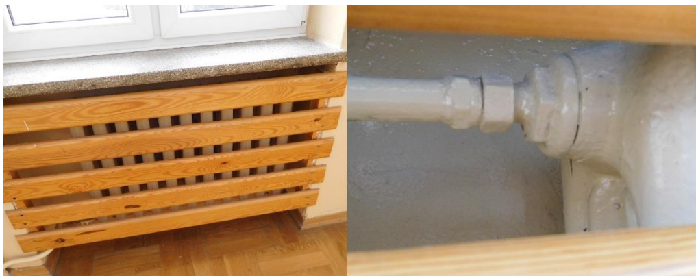
Figure 56 Iron ribbed convectors in corridors
