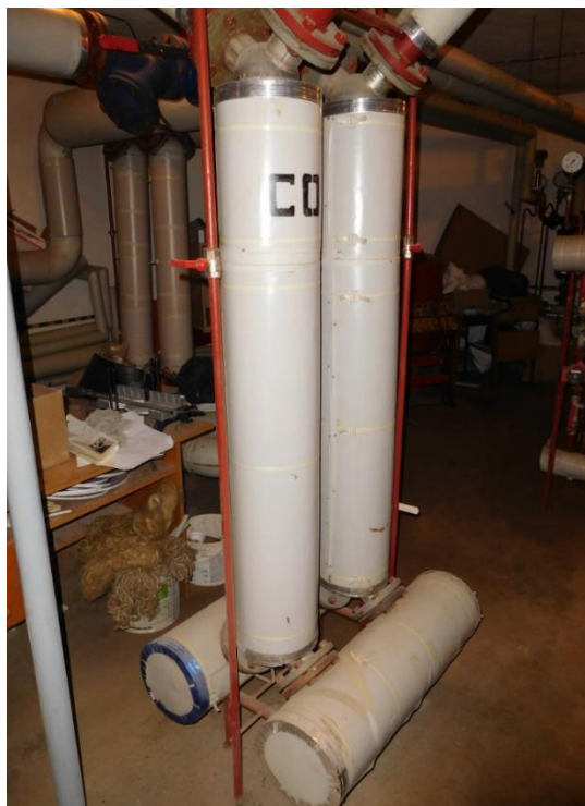
Figure 37 Heating source in the building
