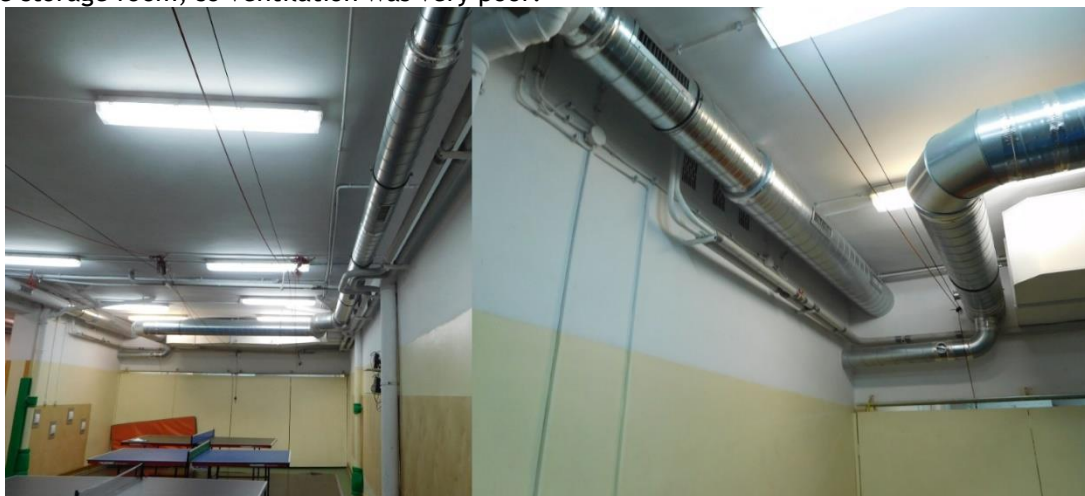
Figure 21 Fencing sport hall ventilation ducts
