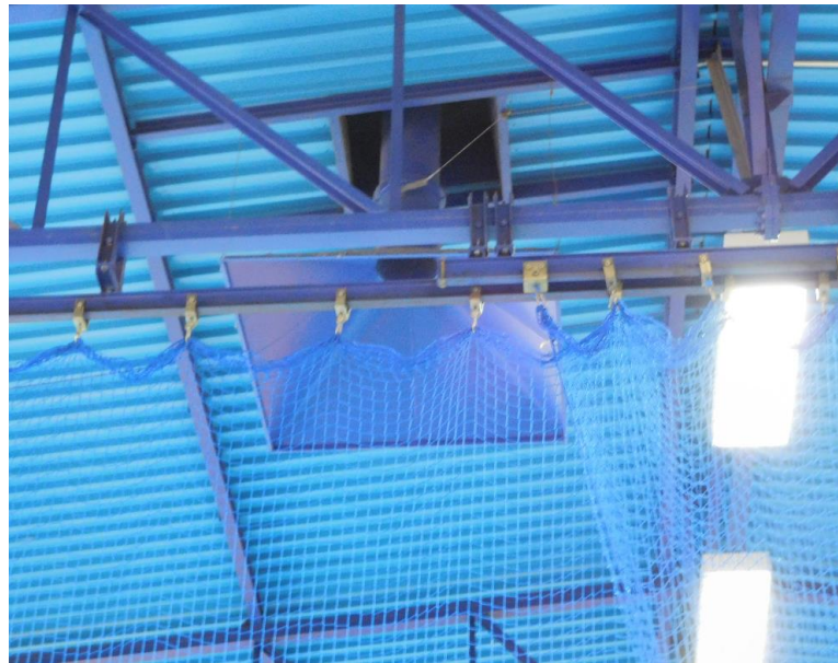
Figure 20 Large sport hall ventilation
