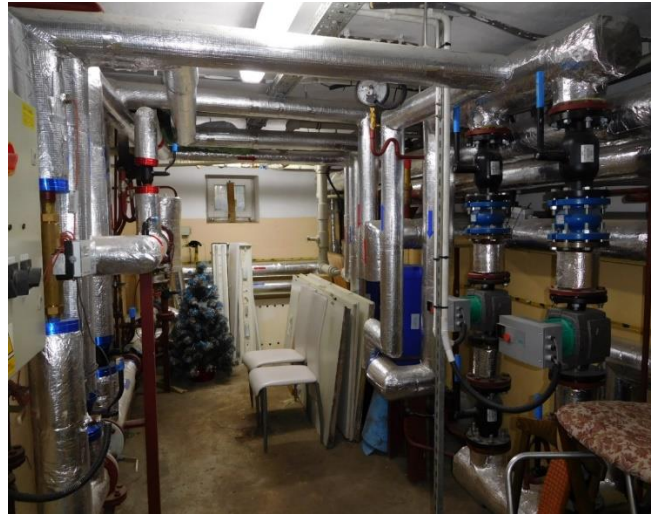
Figure 2 Heating source in the building
