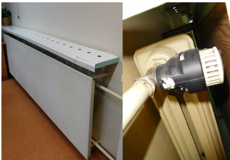
Figure 39 Water convectors with thermostatic valves
