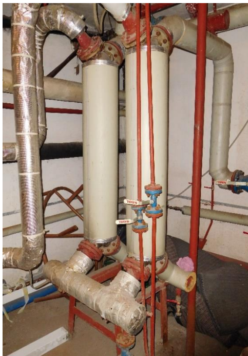
Figure 54 Heating source in the building
