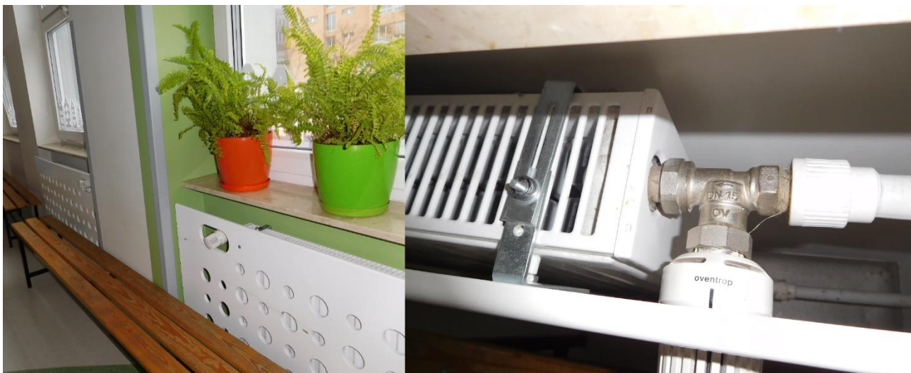
Figure 45 Water convectors with thermostatic valves
