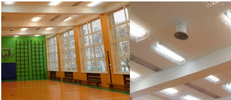
Figure 58 Sport hall ventilation
