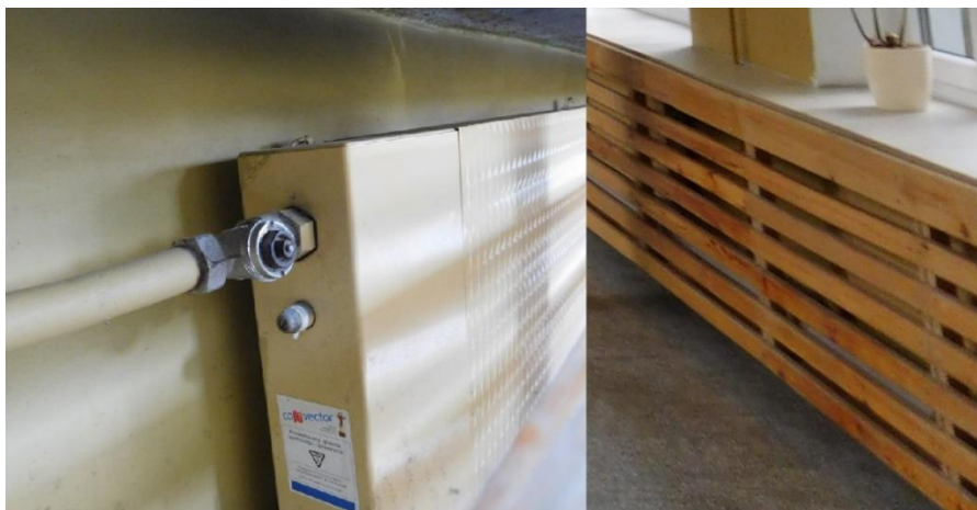
Figure 18 Plate heaters in the building
