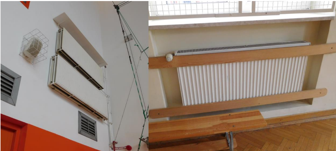
Figure 80 Plate heaters in the sport hall with thermostats
