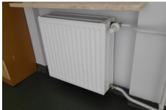
Figure 4 Water convectors with thermostatic valves
