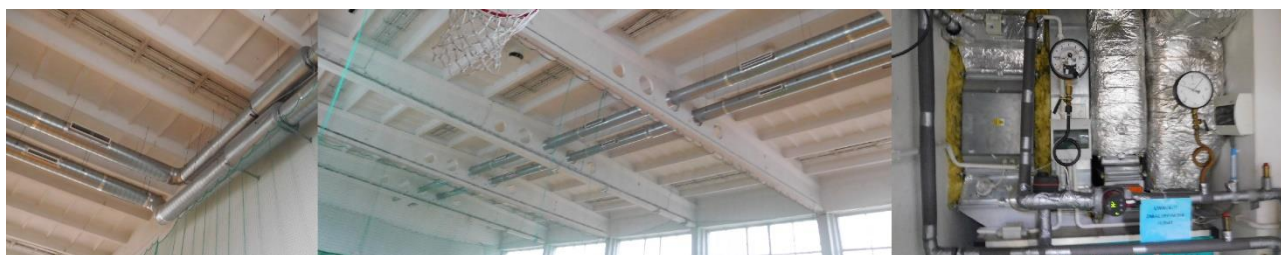
Figure 29 Mechanical ventilation in the sport hall
