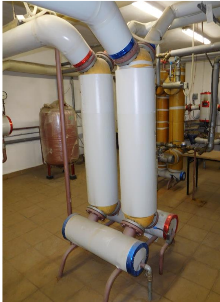
Figure 26 Heating source in the building
