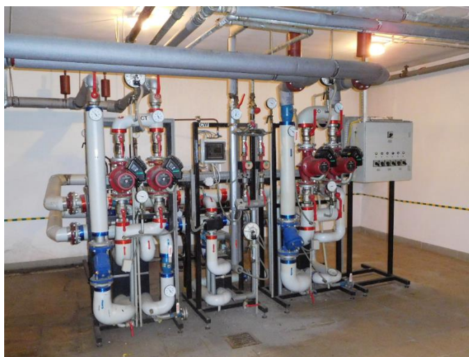
Figure 77 Heating source in the building
