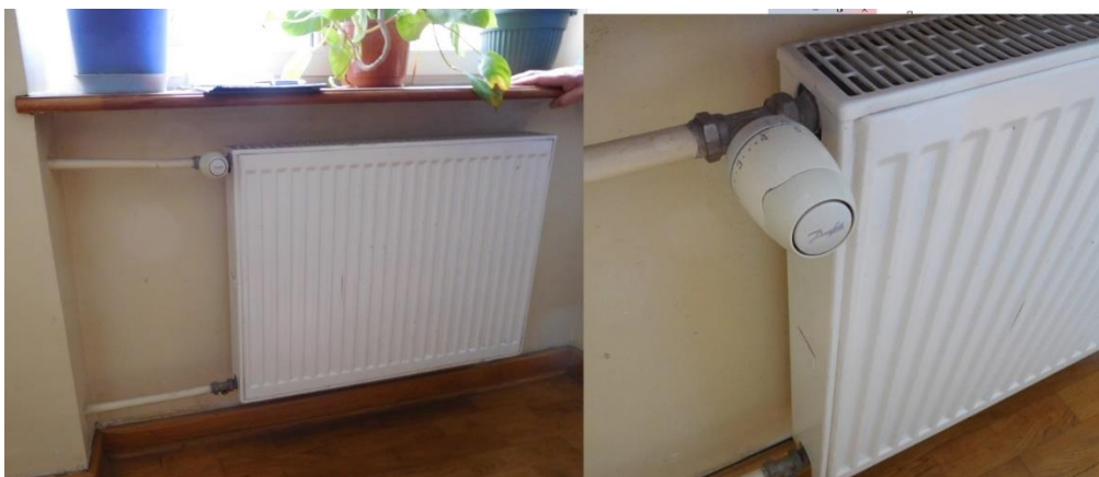
Figure 79 Water convectors with thermostatic valves
